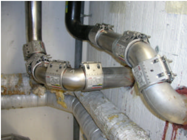
Flexible pipe layout around existing piping
