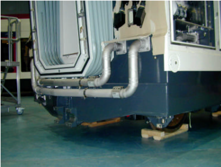
External stainless steel pipe system between tractor and coaches
